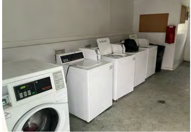
Subject central laundry facility
