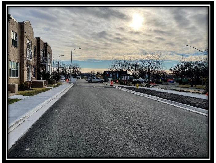
View east on Wood Street showing proposed Block 9 in the right background
