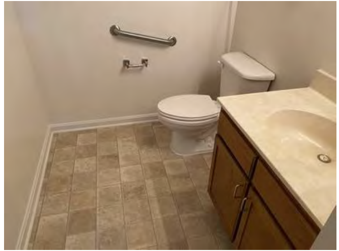
Typical two-bedroom bathroom
