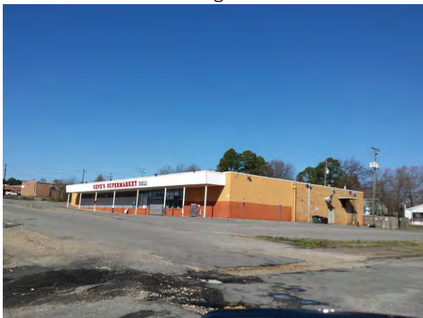
Vacant retail bulding at Bellemeade Road and U.S. Route 1 (Jefferson Davis Highway)
