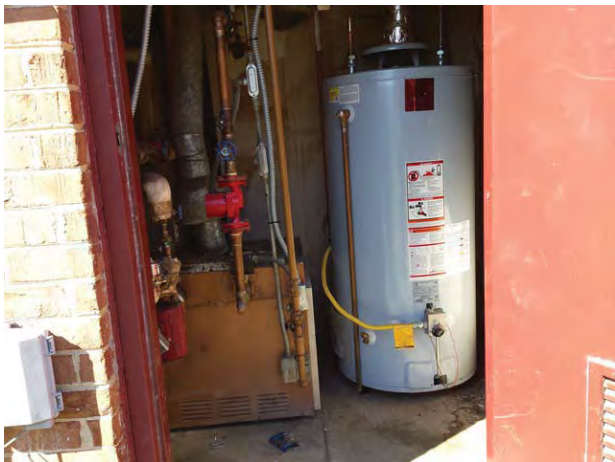
Typical exterior utility closet
