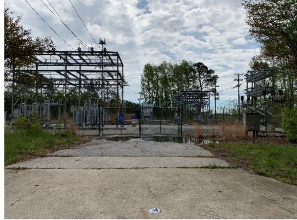
Hodges Ferry Substation
